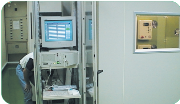
SCADA system for Motor Tester
