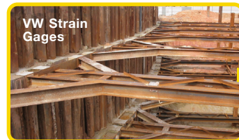
GEOKON VW Load Cell & Arc welded VW Strain Gages
